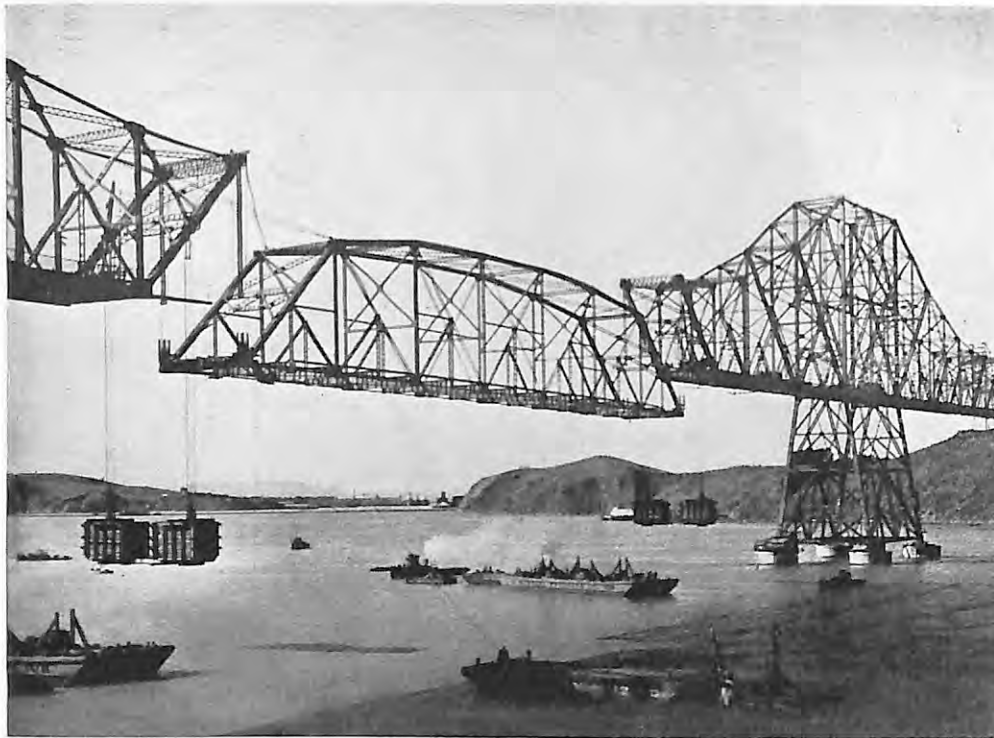
The suspended span of the Carquinez Straights bridge approaching its final position
