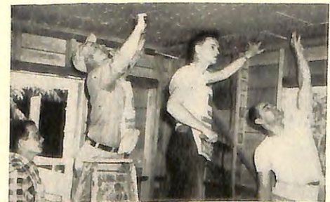
Above: Admiration of the courage of Ray Lambert, blind Banning-Beaumont, Calif., Elk, left, who is building his own home, prompted his fellow Elks to help him. His aides are, left to right: Secy. E. S. Kreitz, E.R. K. B. Husby, Est. Loyal Knight Dan Byerly. An accomplished musician, Mr. Lambert is the lodge Organist.
