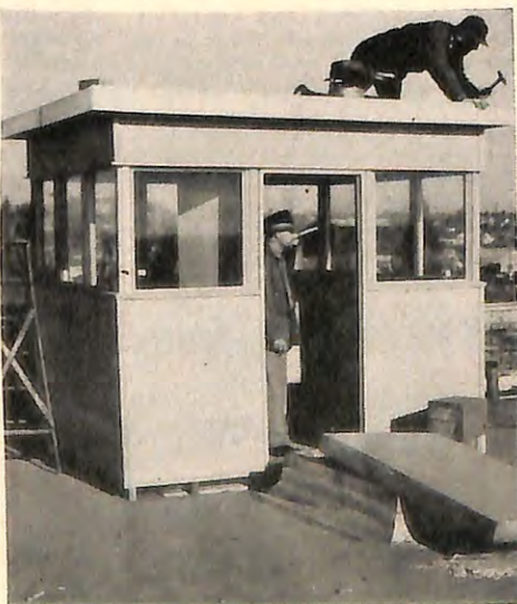
E.R. Dale Phillips of Kalispell, Mont., Lodge was photographed as he inspected the CD ground observation tower atop the lodge building, the tallest in the city which is located near the Canadian border, as one of the volunteers who constructed it puts in a few finishing touches.
