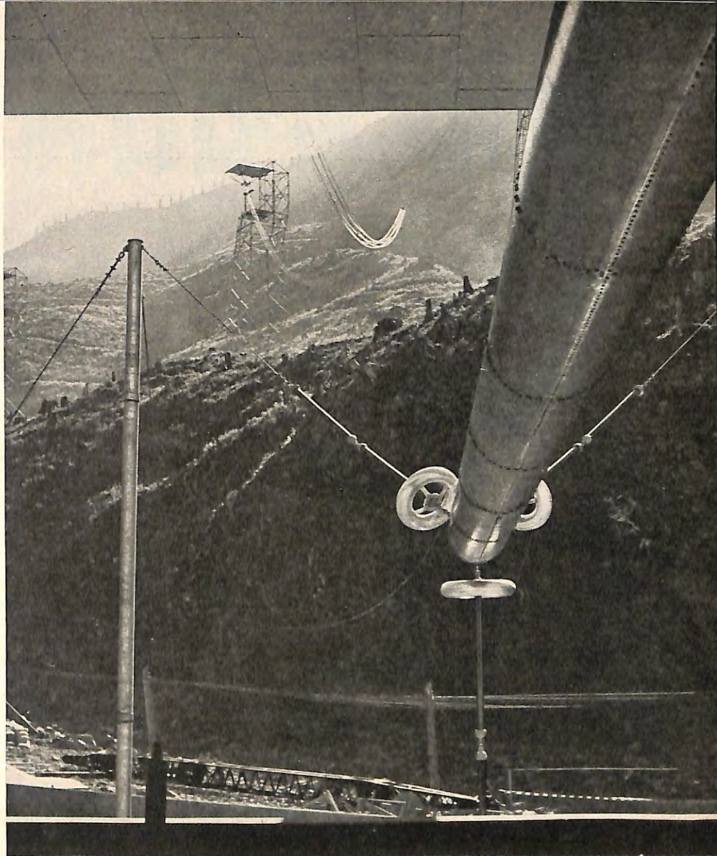
Above: View from transmitter building, along antenna lead-in trunk, shows 145-foot bus tower halfway up the mountain. This is one of thirteen such towers supporting the transmission line.
