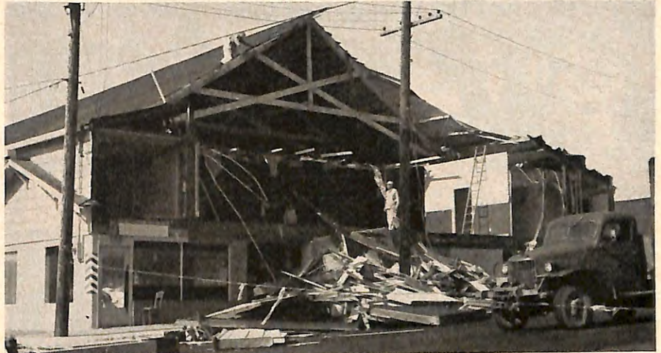
NEWPORT, Oregon, Lodge's home has a lean-to appearance since it suffered severe damage in the Columbus Day storm, the worst in 50 years. Business is going on as usual, however, with temporary cover protecting the damaged area.
