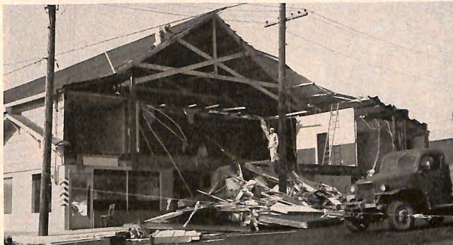
NEWPORT, Oregon, Lodge's home has a lean-to appearance since it suffered severe damage in the Columbus Day storm, the worst in 50 years. Business is going on as usual, however, with temporary cover protecting the damaged area.
