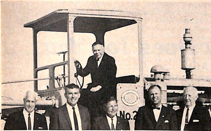
The Grand Exalted Ruler got behind the driver's seat of this grader for groundbreaking ceremonies at Riviera Beach, Fla., Lodge's new home site on Mar. 17. Photographed with him are, l. to r.: Special Deputy Robert Cameron, E.R. Robert Grafton, P.G.E.R. William A. Wall, State Pres. A. C. Van Horn Jr., and Past State Pres. and Grand Lodge Committeeman J. Alex Arnette.
