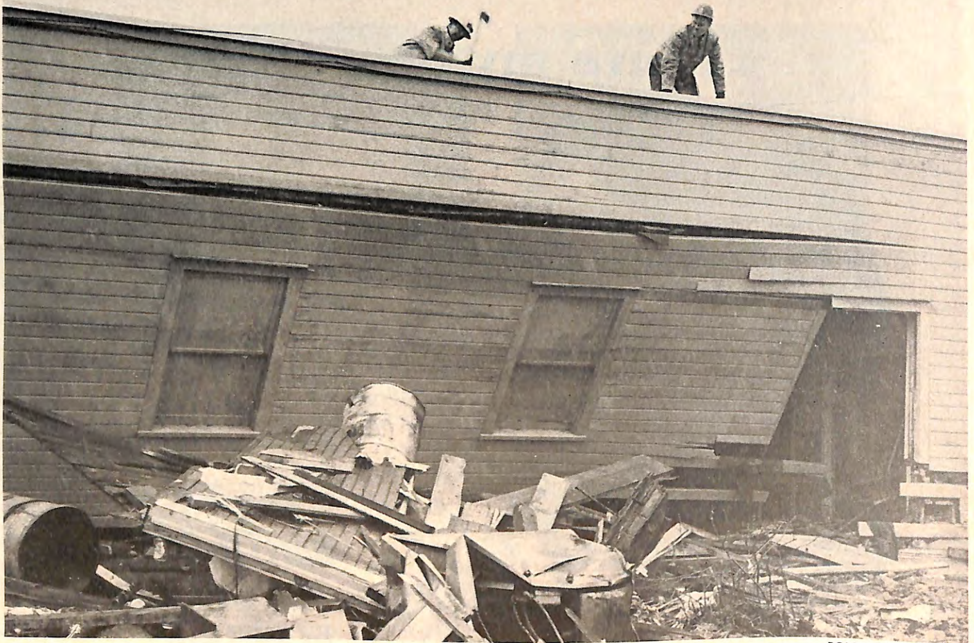
Workmen complete job the 'quake started on Good Friday. Condemned and ordered burned, the home of Kodiak Lodge is a total loss. A car was found in caved-in wall section.
