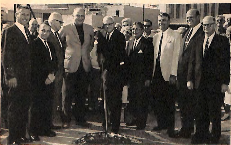
When Fort Lauderdale, Fla., Lodge earlier this year broke ground for the construction of an addition to its home, Grand Exalted Ruler Bush was on the scene. Here he's shown turning the first spade of earth. With Brother Bush are, l. to r., Exalted Ruler Leroy Ludwick; architect Raymond Rood; Mayor Edward Bury of Fort Lauderdale; Florida Assn. President W. S. Compton; Past Grand Exalted Ruler William Wall; District Deputy Robert Grafton; Assn. Vice-Pres. Karl Klaeger; and Frank Adler, Chm. of the Broward County Commission.
