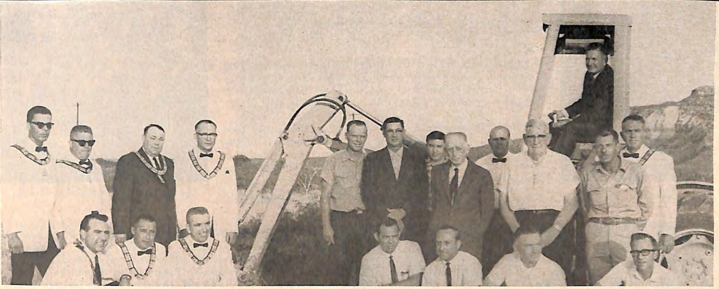
TUCUMCARI, New Mexico, Lodge goes modern with a mechanized ground breaking for its new $200,000 Elks Home and Club. E.R. Bill Potter can be seen in the top row (fourth from left). Mayor Grady Huffman of Tucumcari overlooks from his position aboard the tractor.
