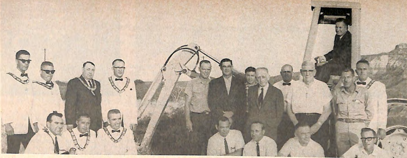
TUCUMCARI, New Mexico, Lodge goes modern with a mechanized ground breaking for its new $200,000 Elks Home and Club. E.R. Bill Potter can be seen in the top row (fourth from left). Mayor Grady Huffman of Tucumcari overlooks from his position aboard the tractor.
