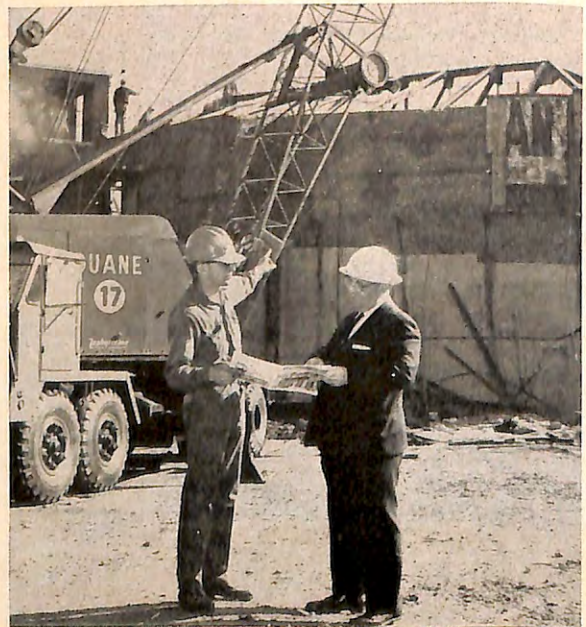
BRIGHTON, Massachusetts, Trustees Chairman Al Basse (right) is shown by engineer George Ross how demolition of an old theater building is progressing. The structure's unused portion was becoming a threat to passersby, so the lodge obtained an order to have the building razed.
