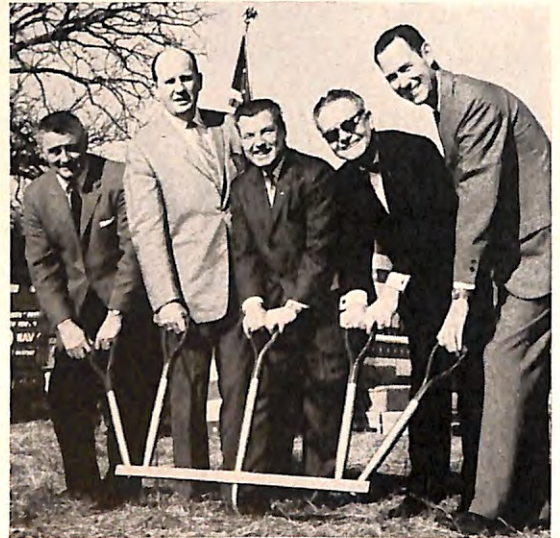
AT ARLINGTON, Texas , ground is broken for a new lodge building. Plans call for a swimming pool, tennis courts, a picnic area, and a baseball diamond, which may be used by Boy and Girl Scouts and Little Leaguers. Moving the first inches of earth are Dan Gould, president of the Arlington Chamber of Commerce; S.P. Joel W. Ellis, Harlingen; E.R. Richard D. Loudon; P.S.P., P.D.D., and Dallas P.E.R. Alex A. McKnight, Arlington, G.L. New Lodge committeeman, and P.E.R. Alvin E. Betzel Jr.
