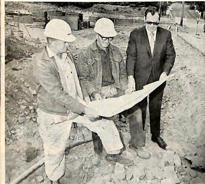
PLANS for a new $115,000 home for Colfax, Wash., Lodge were discussed by Secy. DeLoss Ray (right) and Donald Kaiser and Charles Hollenbeck, builders. Colfax Elks lost their lodge quarters in a fire last January.
