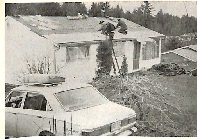
THE ROOF of a local couple's home was repaired recently by Federal Way, Wash., Elks. The Washington State Department of Social and Health Services contacted the lodge that the woman's husband was in the hospital and they didn't have enough money to repair their leaking roof. The lodge raised $100 and formed a work crew to remedy the situation.
