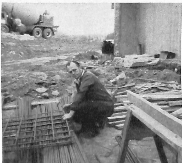
CONSTRUCTION of a $150,000 expansion of the lodge building was begun recently at Sherwood, Ore., Lodge. ER H. Leroy Johnson examined the steel mattings to be used in the structure.
